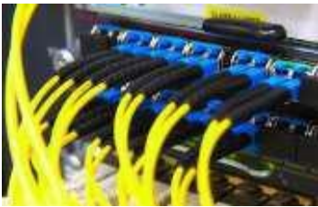
Backbone (Fiber-Optic) Data & Voice cabling
