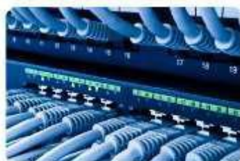
Structured cabling & Cable Management
